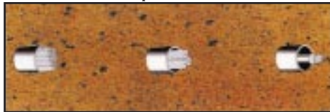
Telephone, Electric Power, and CATV Cables
